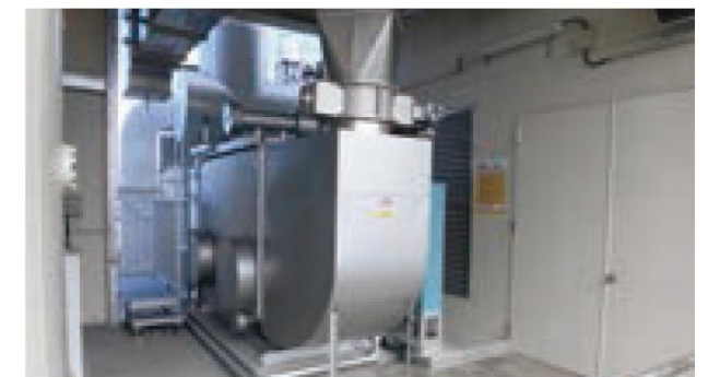
Gumma Works: Exhaust heat recovery boiler
